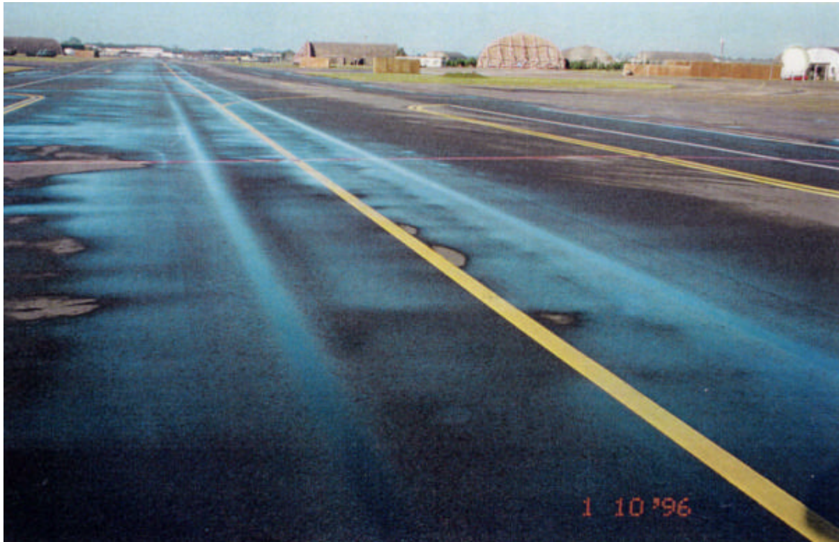
Figure 2. Rutting In Upper Bituminous Layer
