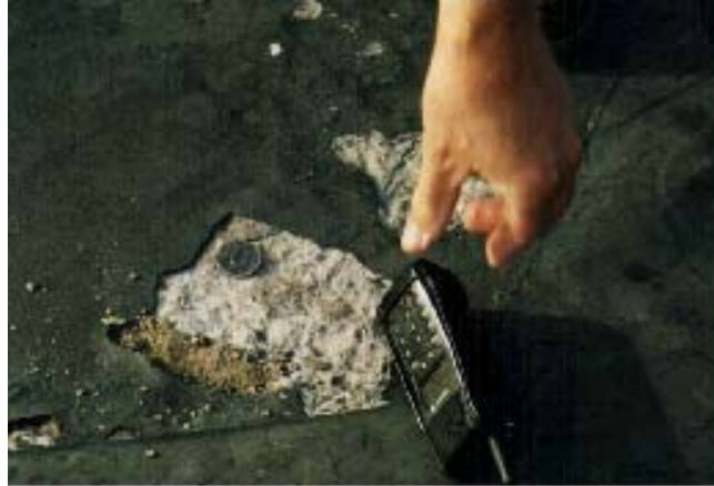
Figure 1. Unsuitable materials for thin concrete layer.
