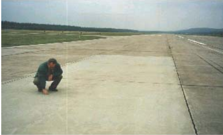
Figure 5. Thin concrete overlay (inlay) Hultsfreds airport done 1994, inspection 1999.
