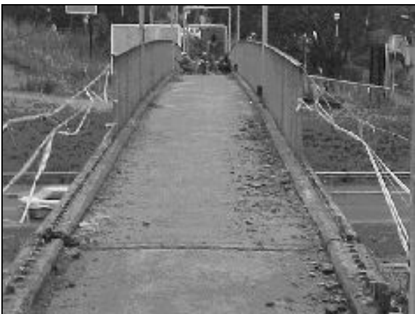
Photograph 1: Stolen pedestrian railings
