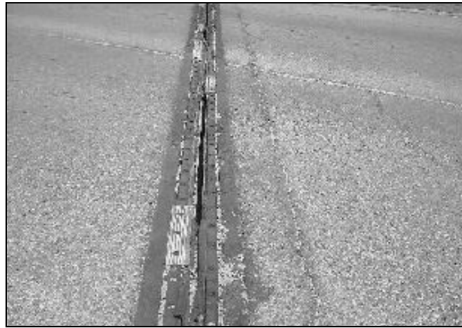
Photograph 3: Theft of aluminium road joint
