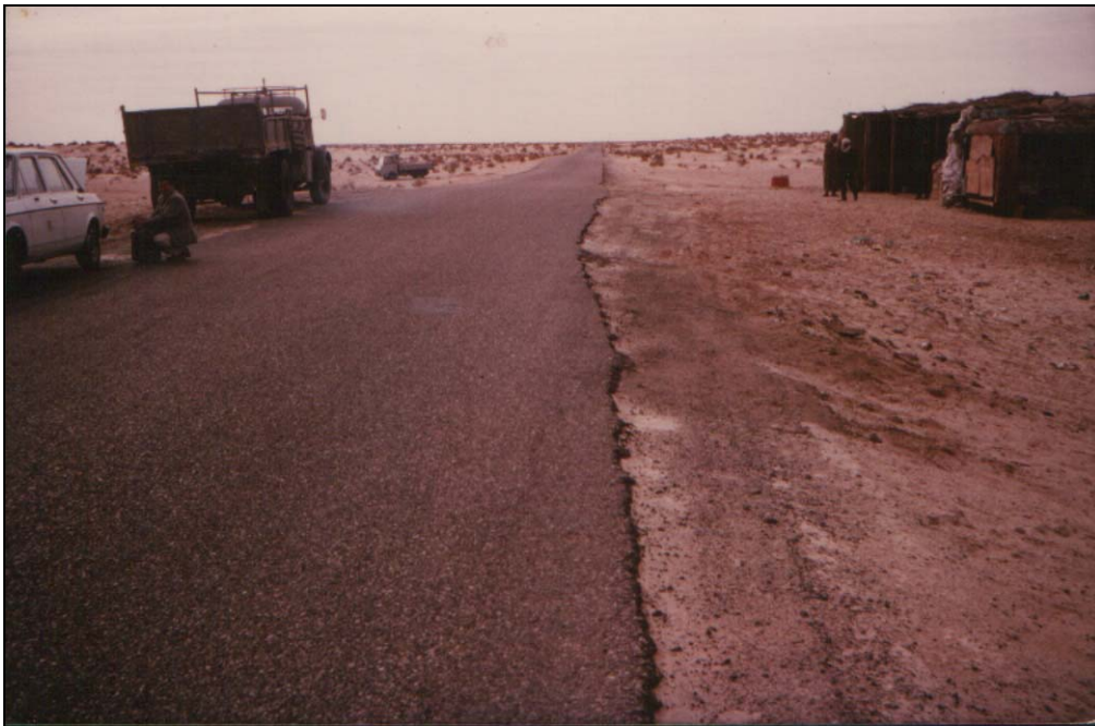
Figure 3: Route Nationale [main road] N° 3 at El Oued: base course gypsum sand with good road setting
