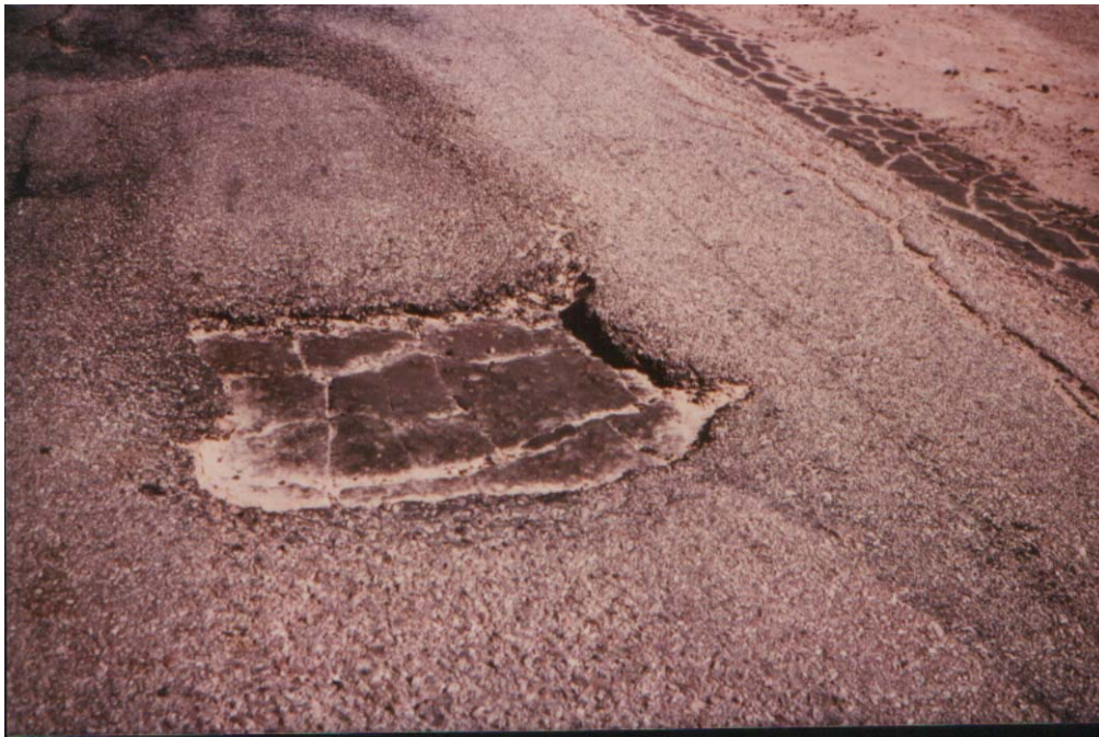
Figure 8 RN 3: Road pavement made of gypsum sands: degradation by cracking
