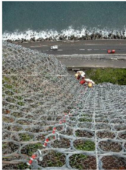
Figure10 - deflecting nets on the road of littoral (P.R.2)
