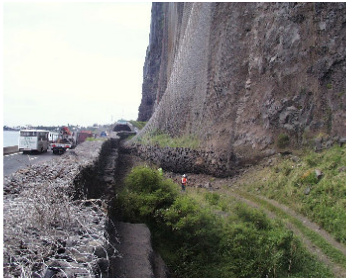
Figure 9 - Crumbling of 500 m 3 on the road of the littoral, April 2003
