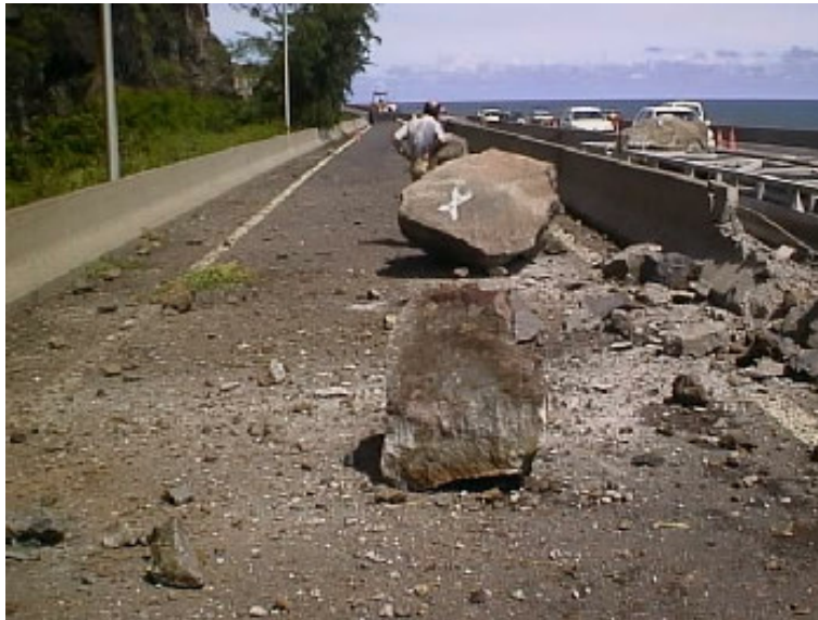
Figure 4 - Fall of blocks on the road of the littoral
