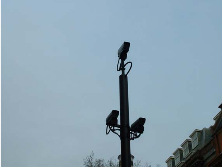
Fig 4 CCTV cameras on entrance to Area
