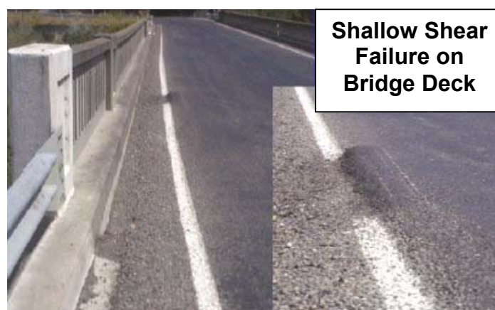
Figure 2 – Evidence of Shallow Shear in Top Surface found on the Highway
