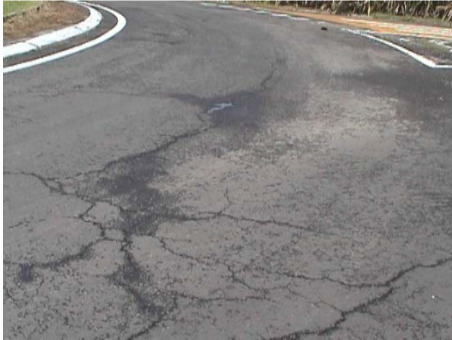
Figure 1 – Cracks and crazing
