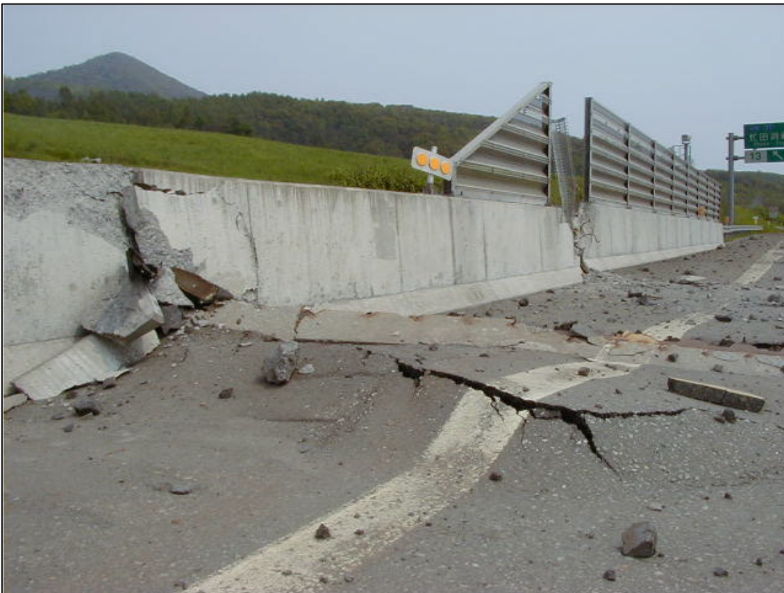
Photo-R.2.2 - Damage to a Bridge
